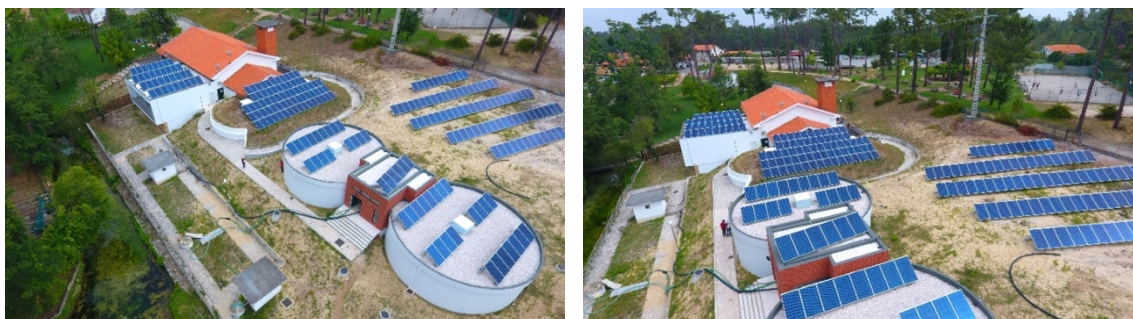
Figure 2 - Solar PV system installed in the water treatment infrastructure of Olhos de Ferverença.
